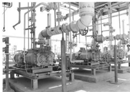
(Left) Bear Clanton, mechanical technician at Sabine River Works, monitoring vacuum pump system. (Above) Busch COBRA dry screw vacuum pump installation at E.I. DuPont, Sabine River Works.
